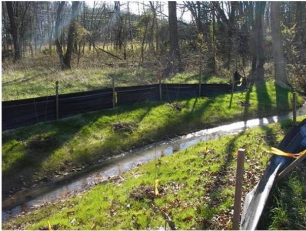
Restored stream channel in Loudoun County following a temporary impact for utility installation
